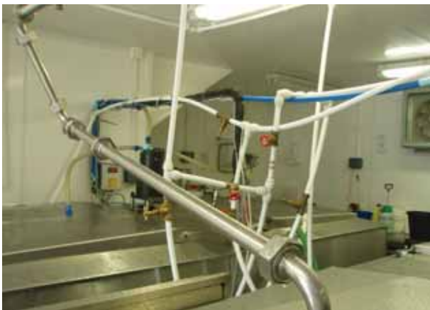
Pipes carrying pumped pasteurised milk into cooling tanks. Source: C.E. Lloyd Swansea University
